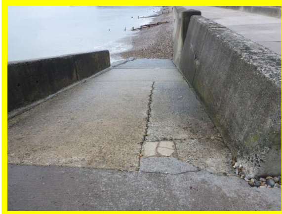
Cracks in deck of access ramp at southern end of promenade (/0102C01) (/0102C01)
