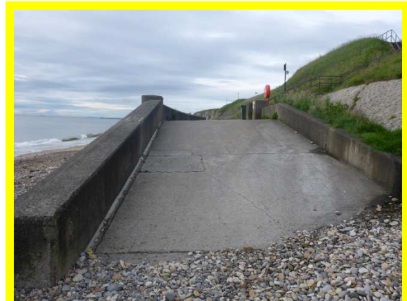
Cracks in deck of access ramp at northern end of promenade (/0102C01)
