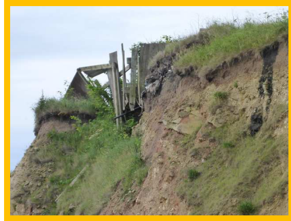
Erosion affecting fence line of properties to south of Dawdon Dene outfall (/0103C01)
