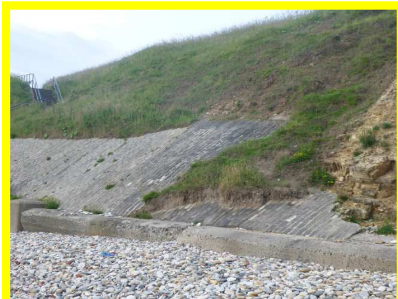
Minor outflanking of blockwork revetment (/0102C01)
