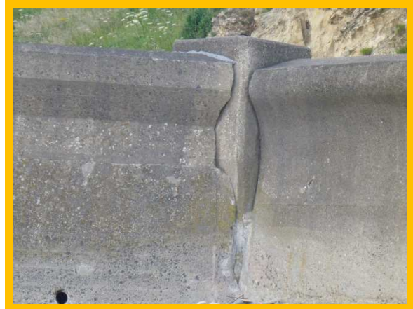
Cracks at junction between sea wall and access steps (/0102C01)
