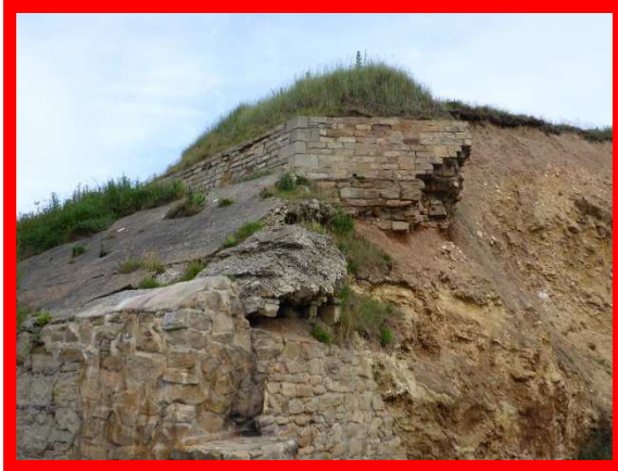
Masonry wall and concrete revetment at tie-in to cliffs breaking-up (/0103C01)
