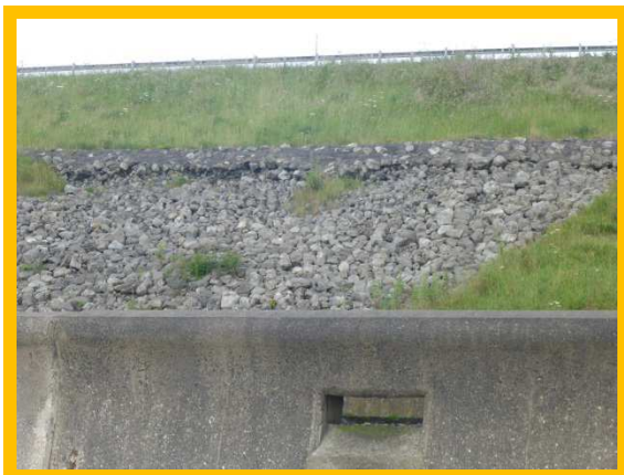
Remedial works needed to 'sunken' area of blockwork revetment (/0102C01)
