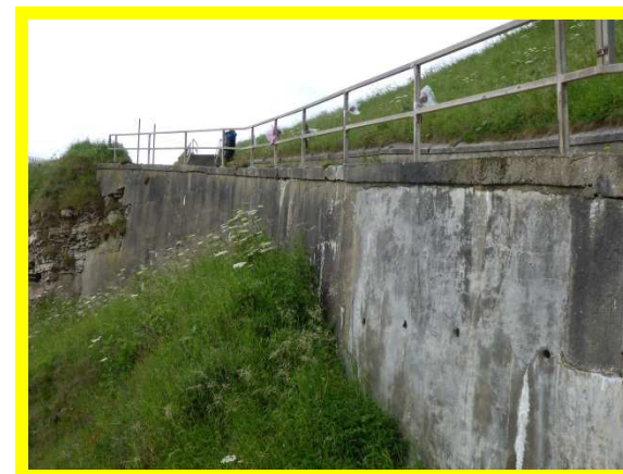
Cracking in retaining wall to access steps and ramp (/0103C07)
