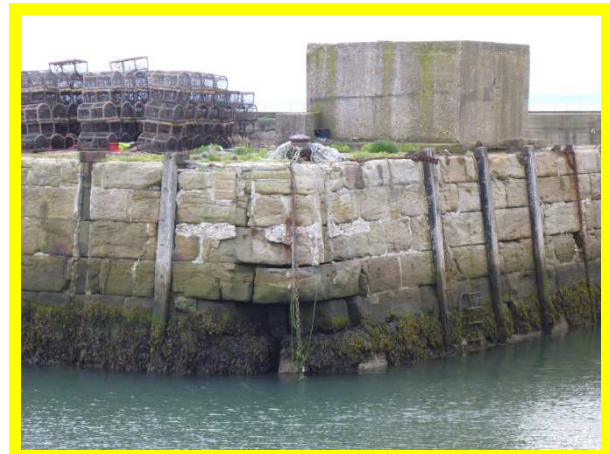
Gaps between blocks at Seaham North Dock (/0104C09)
