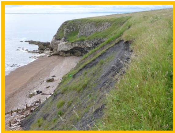
Slippage in cliff at Chemical Beach (/0106C01)
