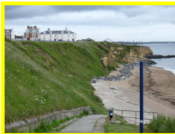
Local slumps in cliffs (/0103C06)
